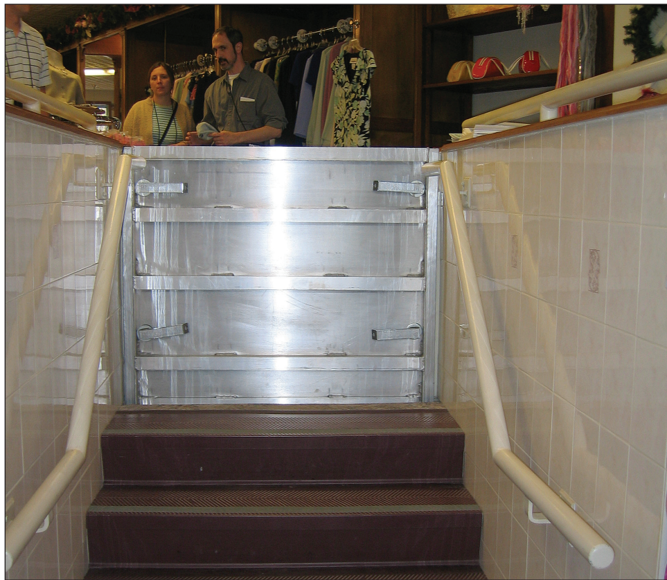
Figure 4-28. Commercial structure in Darlington, WI, mitigated using a combination of wet and dry floodproofing techniques
