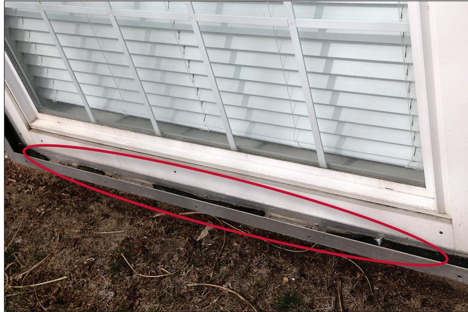
Figure 3-19. A deteriorated flood shield gasket (see red circle) that must be replaced for the shield to seal and function properly (Ocean City, NJ)
