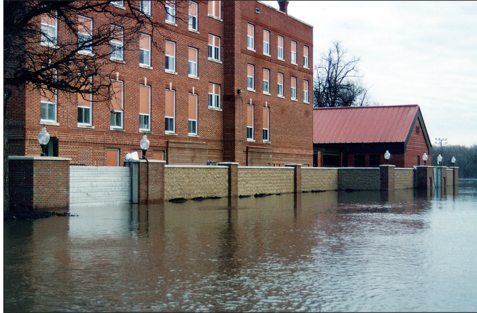
Figure 4-1. Typical masonry floodwall with engineered closures, which protected the Oak Grove Lutheran School in Fargo, ND, from flooding in 2001 (source: Flood Control America, LLC)
